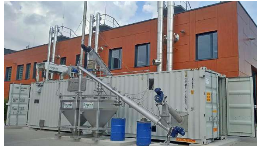
Pyrolysis plant REW Regenis, Quakenbrück [2]
